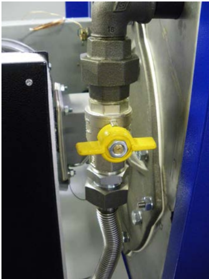
Figure 8.1.1 - Gas Isolating Valve
