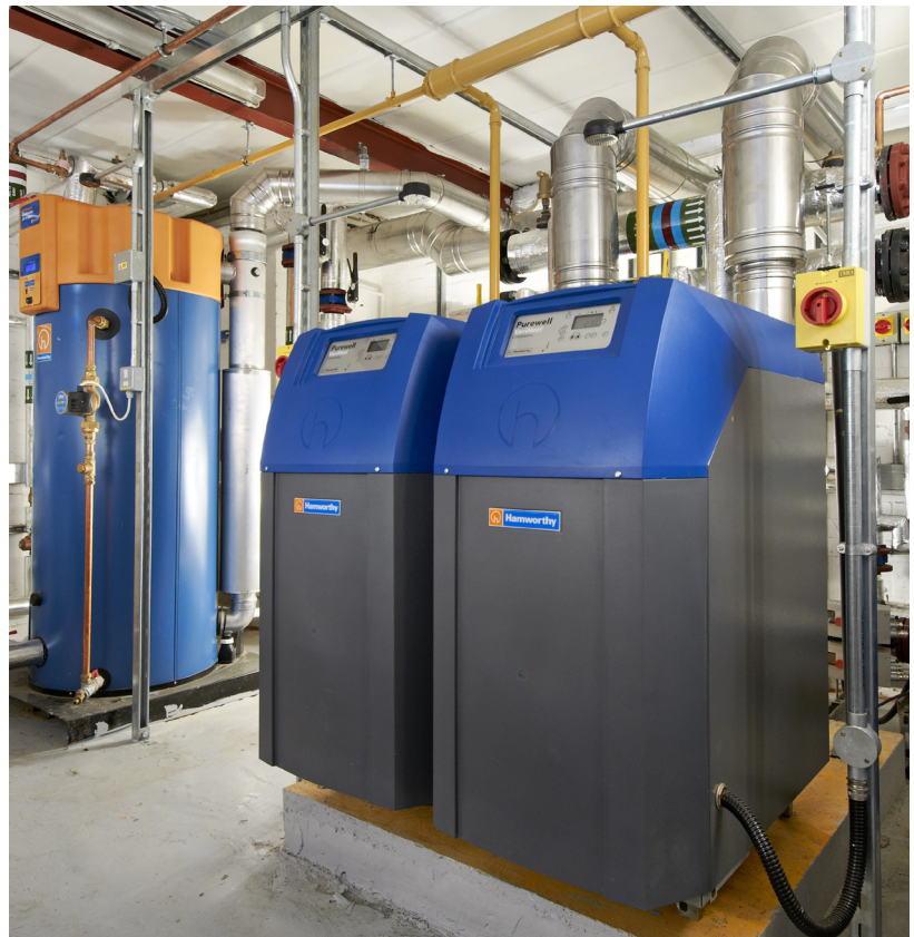
Typical plant room with Purewell VariHeat c highly efficient condensing boilers and a Dorchester DR-FC Evo condensing water heater.
