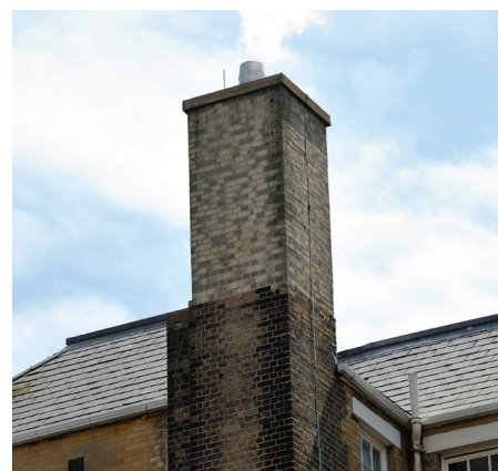
The existing chimney was lined to enable it to cope with condensate
