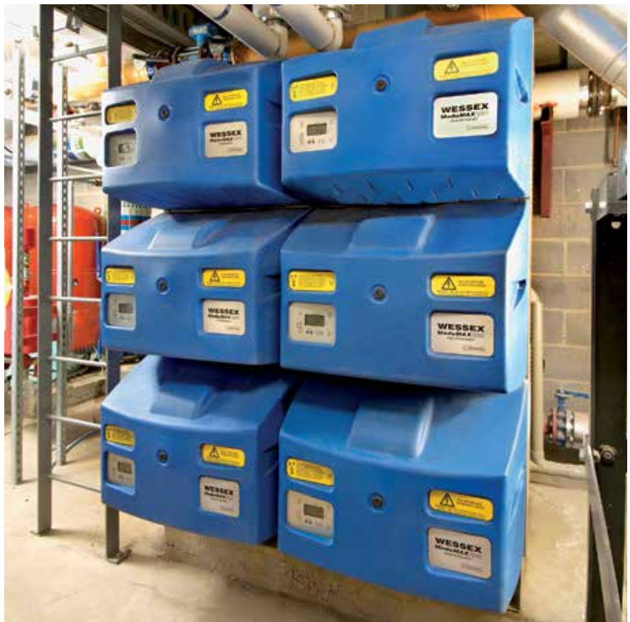
Two Wessex ModuMax 250/750c boilers with a total output of 1500kW.
