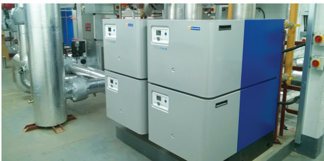
Two Wessex ModuMax mk3 WM254/508V boilers now heat the whole cathedral up within one day, compared to a week by the previous boilers.
