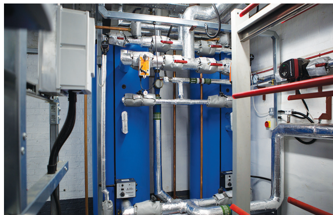
Two Powerstock PS500 calorifiers provide DHW for the cathedral.
