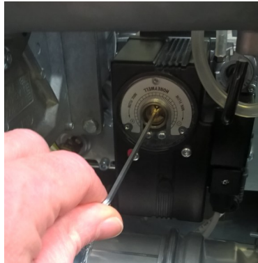
Figure 8.6.4 - Adjusting gas valve throttle
